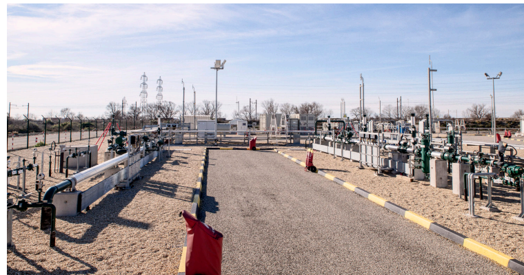
Hydrogen is injected in the grid since 02 2020
